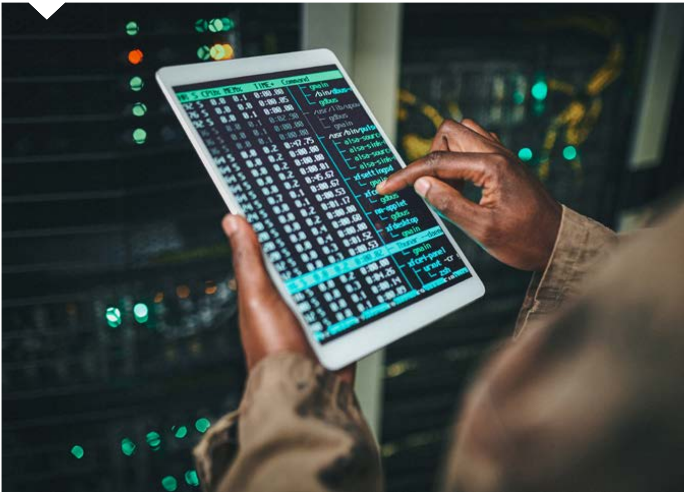
Running the diagnostics using a tablet in a server room
