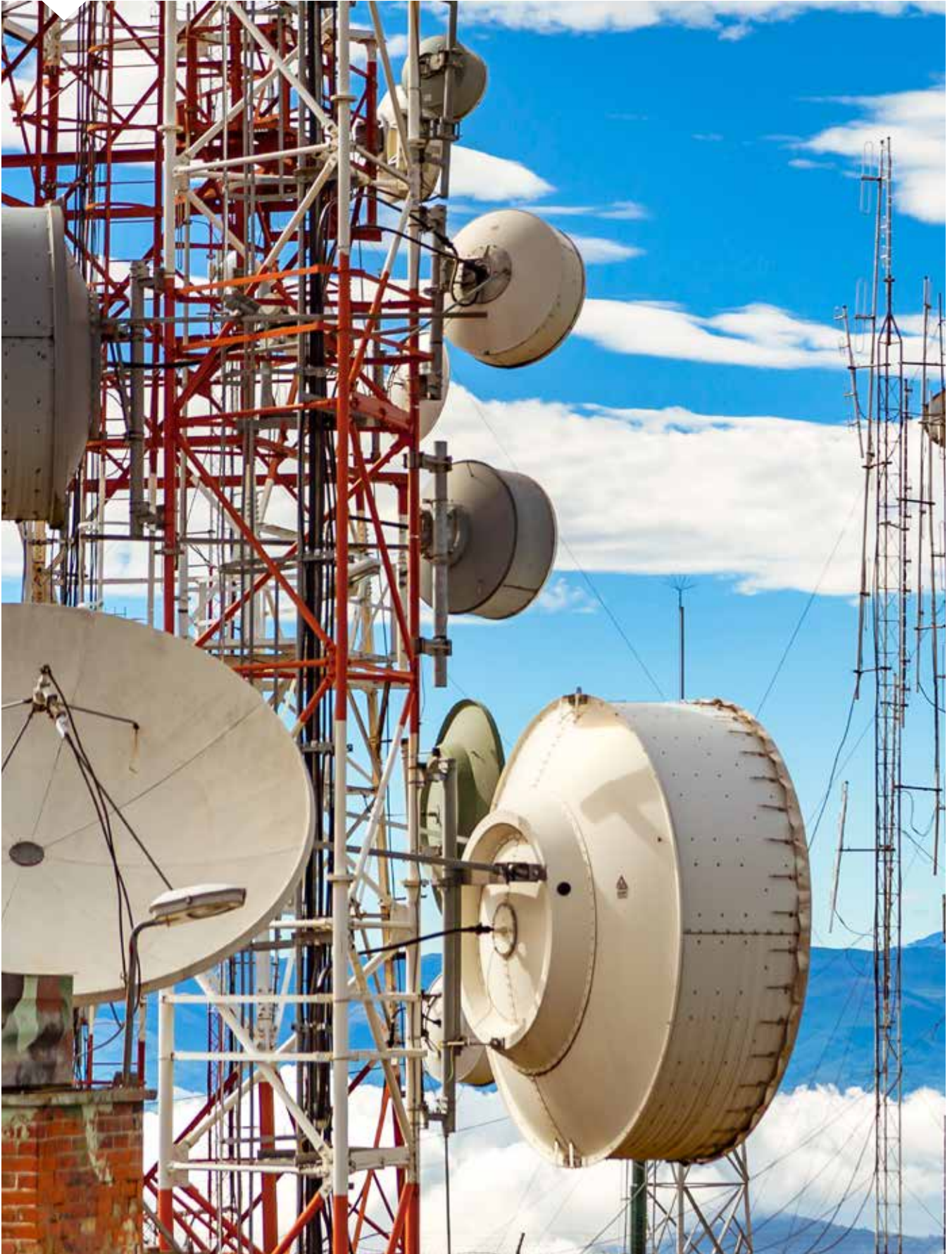
Telecom antennas above the city of Quito, Ecuador
