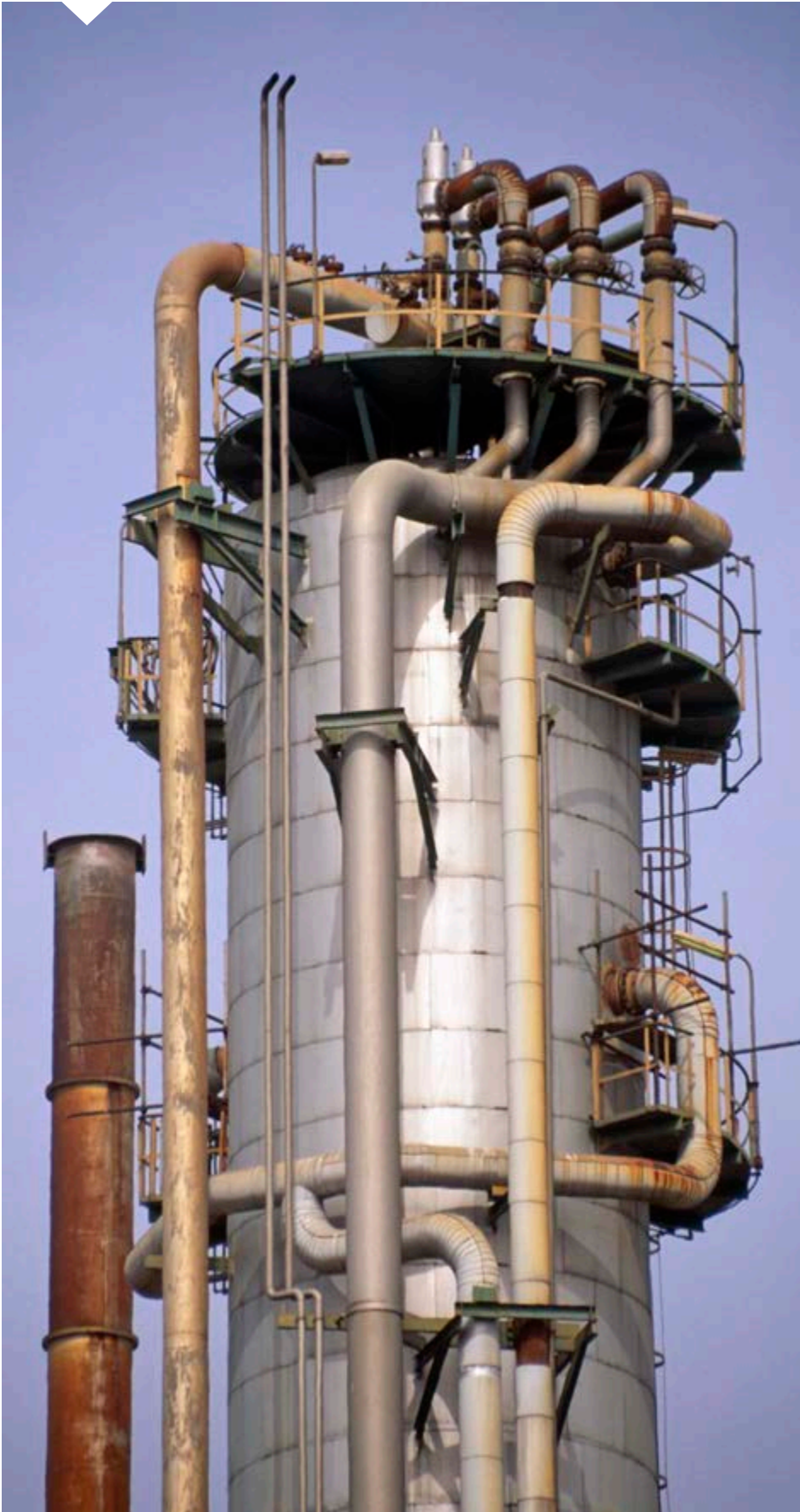
Top of distillation column, Nigeria, Kaduna, NNPC
