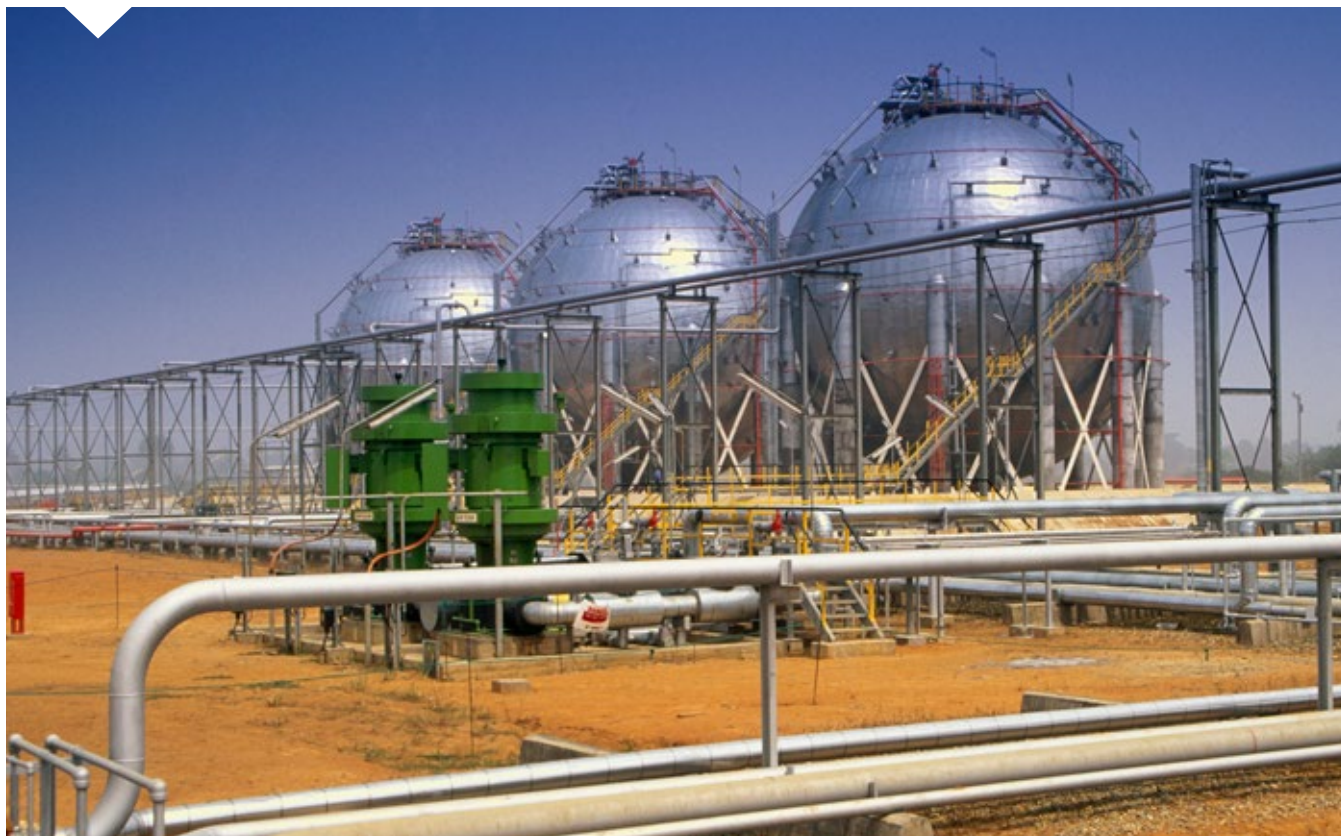
Oil storage tank with feed pipes leading to power station boilers, Nigeria, Africa
